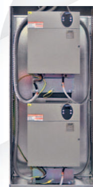
Frequency drive Inverter
